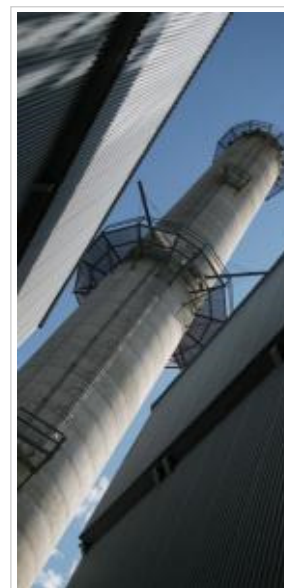
The cogeneration facility's smokestack rises into the sky. But you won't see any smoke coming out of it. DTH/Lauren McCay
